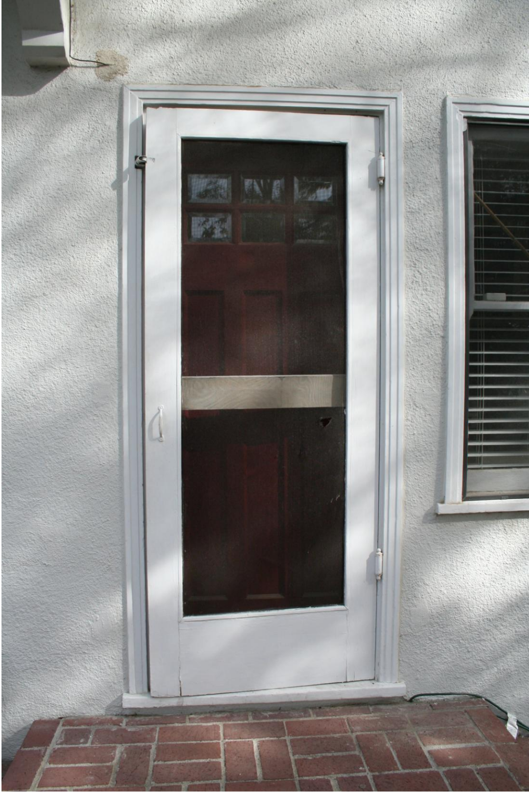
Photograph 16: View of the west elevation side entry with its original paneled wood Craftsman style lighted door.
