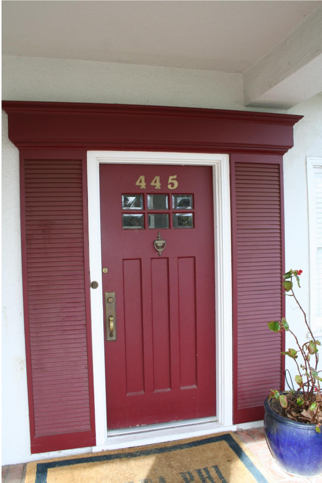
Photograph 17: Close-up of the original paneled wood and lighted Craftsman front entry door with later louvered surrounds and crown.
