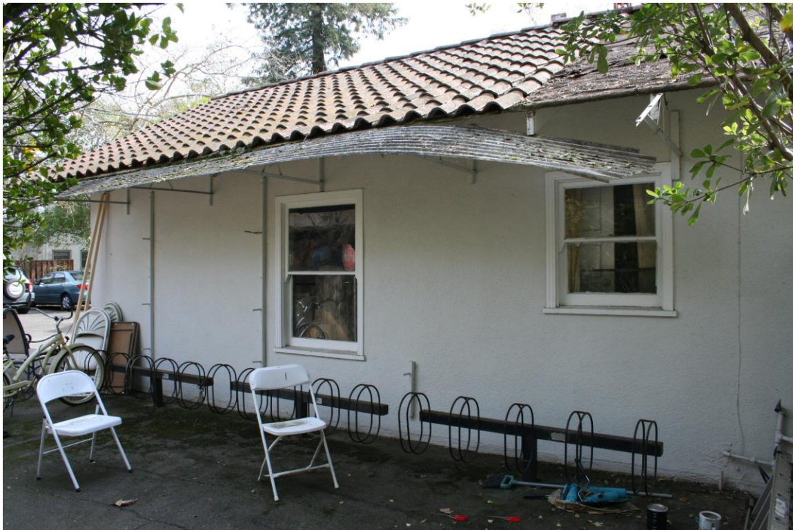
Photograph 12: View of the north elevation of the two-car garage, looking southeast. Note the original wood-sash, double-hung windows. The wood cover is a later addition to keep the rain from the bike rack.
