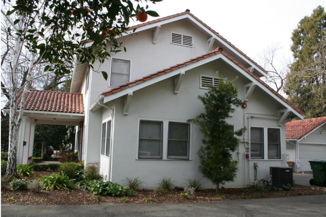
Photograph 5: View of the east elevation of the residence with original double-hung, wood-sash windows, and knee braces under the roof eaves.
