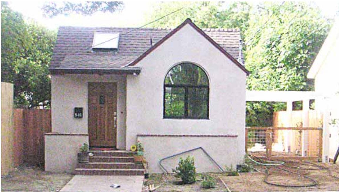
Poulos added a second unit behind 539 in 206-7. Here it is near completion.
